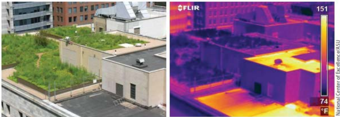
Figure 2 Temperature differences between a Green and Conventional Roof. Green roof is almost 40 °C cooler than the neighboring conventional roof
